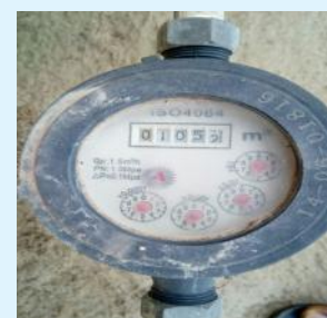
Domestic water meter in installed in Kumasi by Ghana Water Company Limited.
